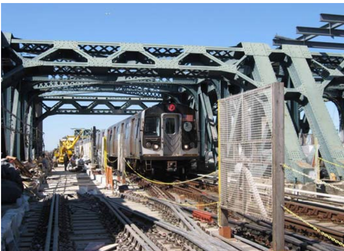
Just north of the Fourth Avenue station, a southbound F train led by Alstom R-160A 9773 is about to stop at the temporary platform. Notice that the fourth switch of this double crossover has yet to be installed.
