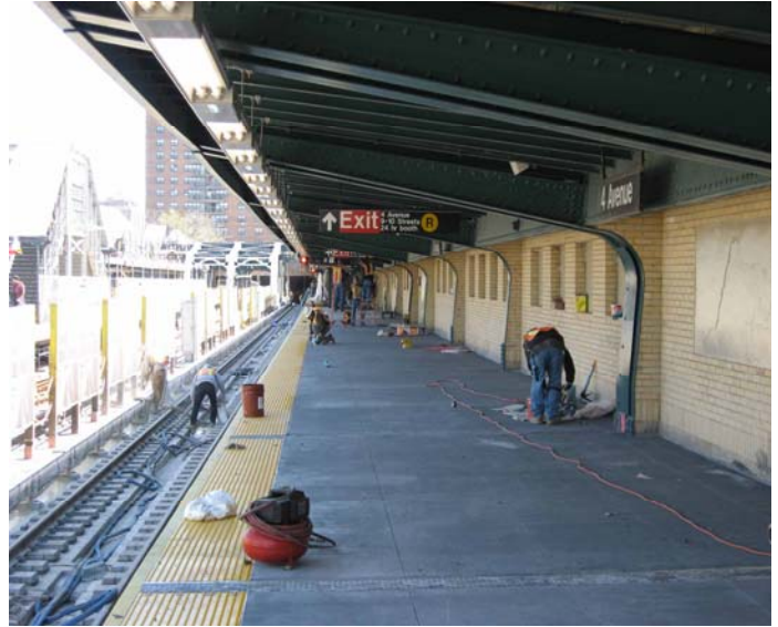
Contractors busy at work putting the finishing touches on the southbound platform at Fourth Avenue.
