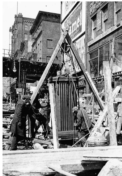
Whitehall Street station under construction: transformer being lowered into subway. Bernard Linder collection
