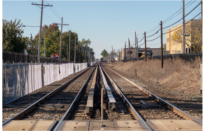
View west from the Covert Avenue grade crossing in New Hyde Park on October 25, 2018. This is the westernmost grade crossing in the project area and will be replaced with an underpass. Construction barrier fencing has been installed along most of the right-of-way between Floral Park and Hicksville on the south side of existing Track 2, which is where the new third track will be built.
