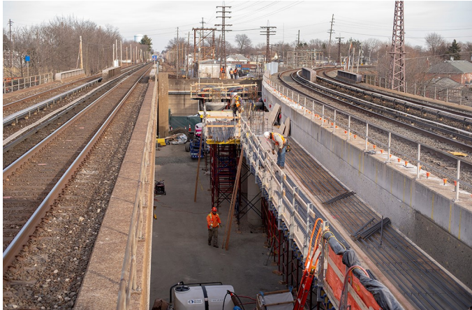
In this view from January 15, 2019, the new support columns have already been poured for the new track connection from the existing westward Hempstead Branch Track 1 (just to the right of the workers) to the new third track. In a bow to the architectural style of the existing elevated structure, these new columns exactly match those dating from 1962, when Floral Park was grade-separated.
