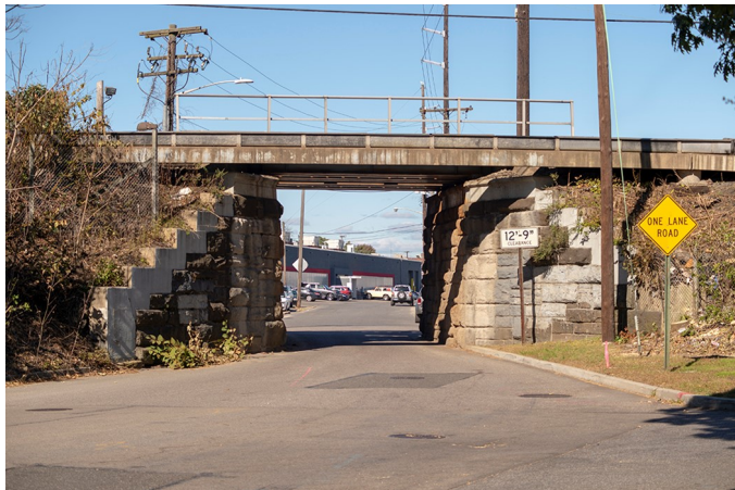
Located midway between the New Hyde Park and Merillon Avenue stations at milepost 16.96, the Denton Avenue bridge was constructed in 1889 and was rebuilt at some point in the last century. You can see that the original stone abutments were added to with a concrete layer. The bridge deck is supposed to be completely rebuilt for three tracks but not, surprisingly, widened. The existing stone abutments are supposed to be extended to accommodate the third track and a traffic light will be installed to control vehicular traffic through the "one-lane" underpass. Photo taken on October 25, 2018. Technically, three-quarters of this bridge is located in the incorporated village of Garden City and one-quarter in North New Hyde Park (a census-designated place).
