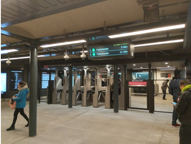
28 St 6 , reopened 1/14/2019, showing the fare array, LED lighting, non-full height gates, and new-style countdown clock display.
