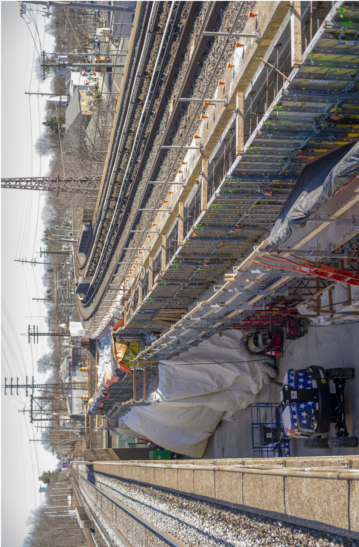
LIRR Main Line Third Track project continues moving forward. Looking east from the center platform of Floral Park station (east of Tulip Avenue) on 2/9/2019. This is the modification of the viaduct for the third track, which will include new bridges over South Tyson Avenue (the bridge in the near distance) and Plainfield Avenue (beyond the station in the distance).
