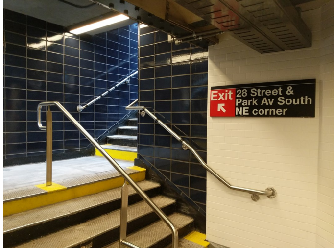
Street stairs leading from the northbound platform at 28 St 6 , showing new tile work, railings, stair treads, and LED lighting.
