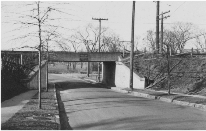
A little east of the Malba station was the Malba Drive undergrade bridge. Built in 1908, this was one of the very few concrete structures on the branch; 3/3/1932.
