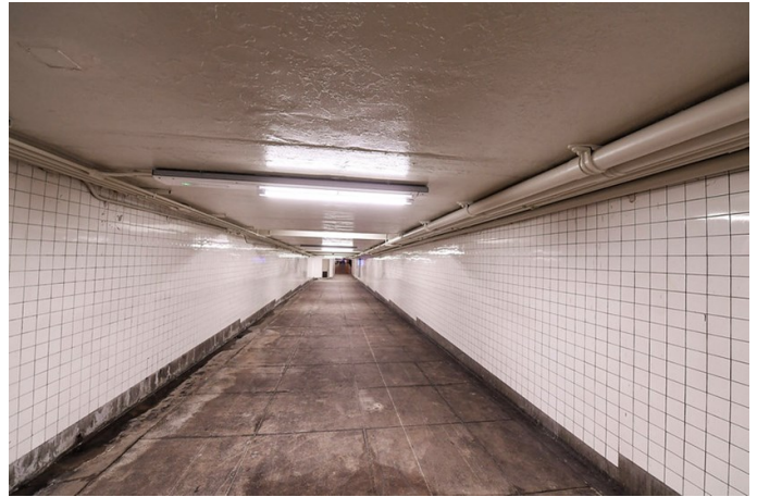
Looking east down the passageway to the Manhattan-bound platform from the mezzanine.
