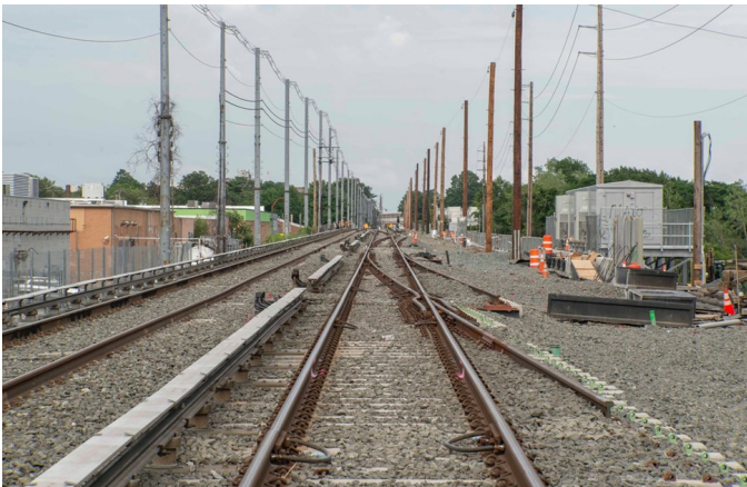
The view looking east at the middle of the new Nassau 1 Interlocking on July 11, 2020. You can see that the two crossovers to what will be the new eastbound local track (future Track 2, to the right) are only partially installed.
