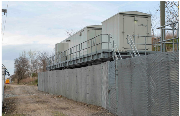
This is an example of one of the new Central Instrument Rooms located along the Long Beach Branch right-of-way that house most of the new signal equipment. As you can see, it is mounted quite high up off the ground. This particular location houses the relays, etc. that control Lead Interlocking, at the end of double track, and is only about 325 feet away from the water's edge of Reynolds Channel. View northwest on April 14.
