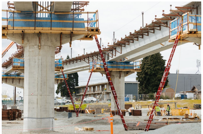
The first girders are going up at the future Kent/Des Moines station. Sound Transit photograph
