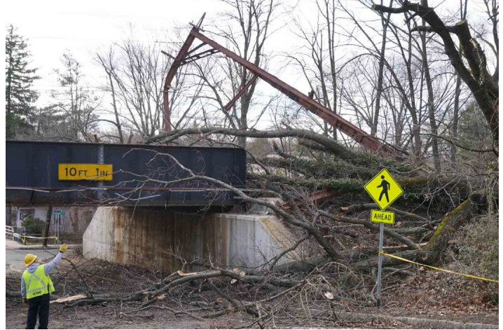
Downed catenary support near Maplewood. NJTransit photo
