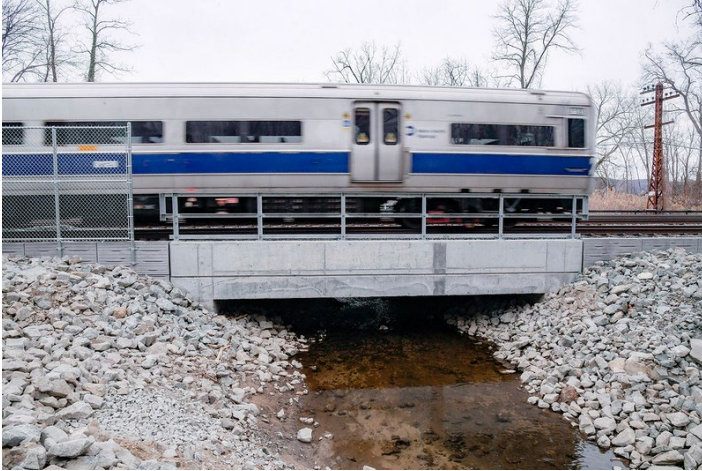
Looking west at the new culvert over Wickers Creek in Dobbs Ferry on the Hudson Line. Marc A. Hermann photo
