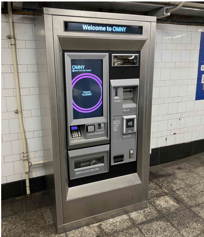
One of the recently-installed OMNY vending machines, as seen on June 3. This one is located on the BMT Brighton Line at the Atlantic Avenue-Barclays Center Station in Fare Control Area B2 (at the bottom of the stairway leading to the LIRR's Tracks 1 and 2). Jeff Erlitz photo
