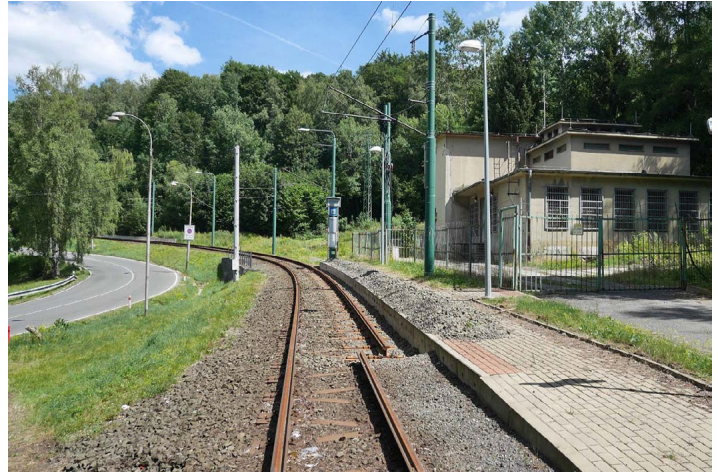
Looking almost due north at the rebuilt Měnirna tram stop, three stops from the terminal in Jablonec nad Nisou on July 28, 2022 during the reconstruction and re-gauging of the line. Before the rebuild, this tram stop was to the photographer’s back.
